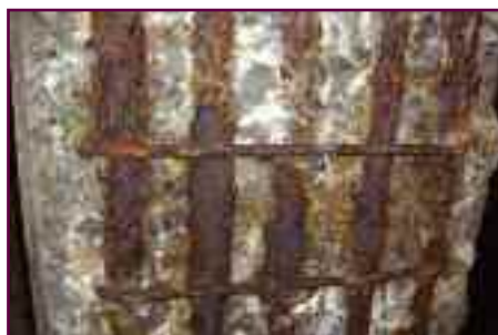
Figure 1: Concrete cover spalling due to reinforcement corrosion.
