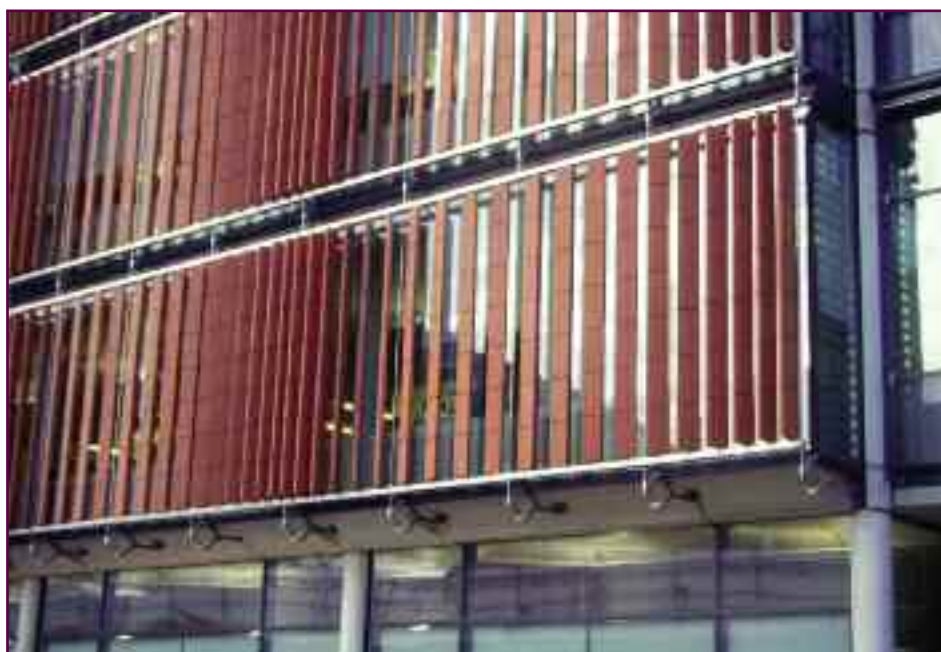
(Top) Means of access for cleaning and maintenance must be considered during the early design stage. (Above) External shading devices can come in many configurations.
