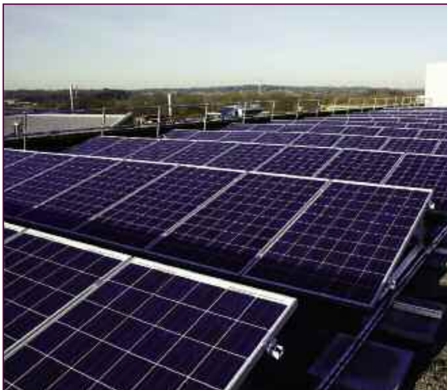
(Top) Low Power Applications such as LED Lighting are becoming more prevalent in buildings. (Above) Trial installation of the University of Strathclyde Project at BRE Watford.
