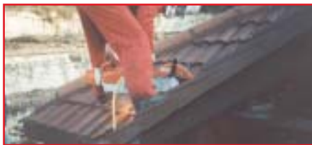
(Top) A circular saw generating dust when cutting roof tiles. (Above) the same circular saw using a water spray when cutting tiles.
