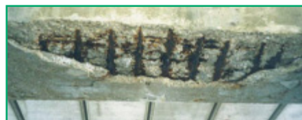
An example of advanced concrete corrosion
