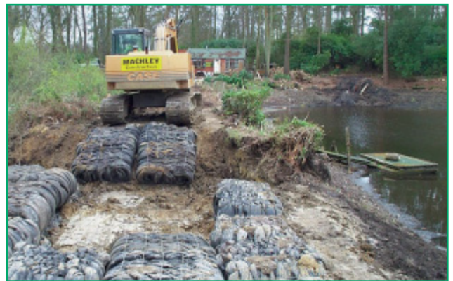
Enviro-Block tyre bales in use as part of an embankment dam (Photo courtesy of Anglo Environmental and Mackley Construction)
